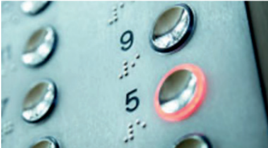
Lift control buttons suitable for many users with: contrasting fonts, lit buttons and braille to indicate the different floor stops.
